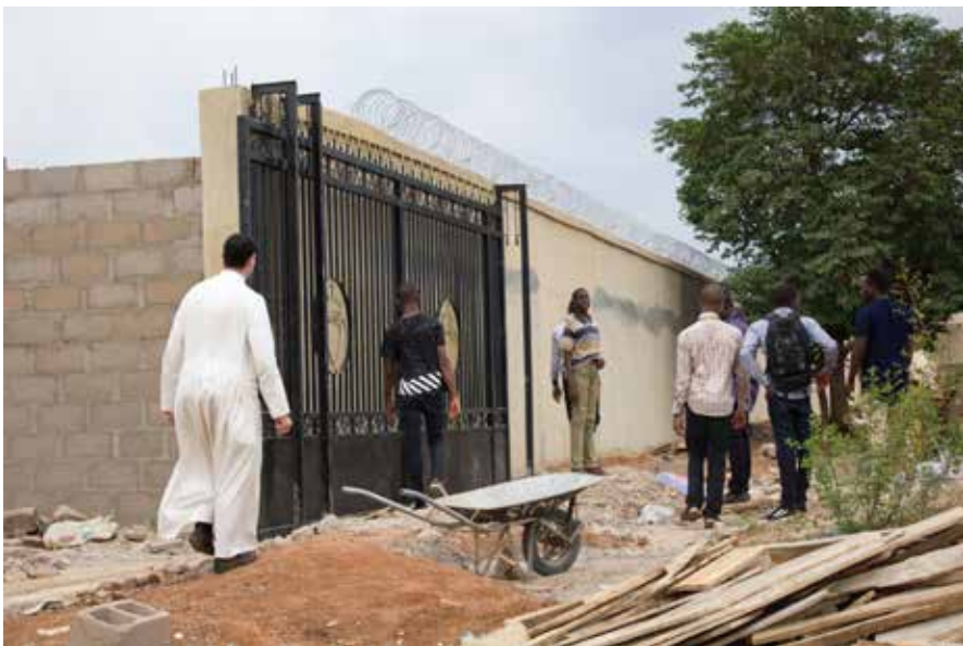
Inspection of the work on the gate and the wall by Father Benedict
